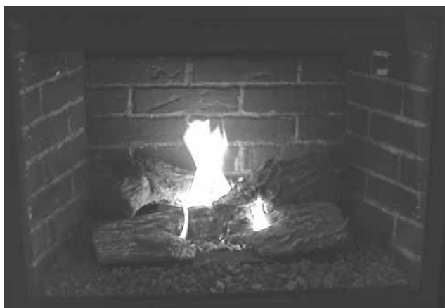
Figure 51 - Burner Flame Appearance Model SLDVT-30 and 35
