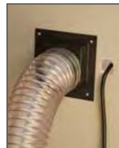
4" universal dust port on the cabinet pulls away the bulk of chips and sawdust.
