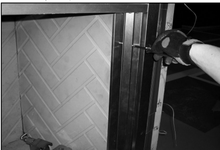
Figure 6.3 Loosen Refractory Retaining Strip
