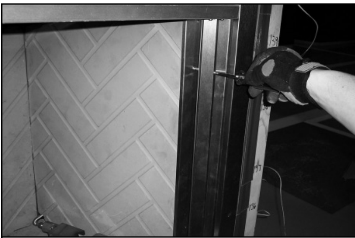
Figure 12.3 Loosen Refractory Retaining Strip
