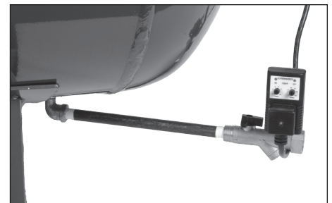
Figure 17 - Automatic Tank Drain
