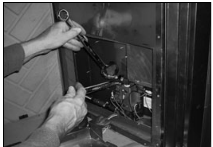
Figure 12.6 Turn off Gas Valve
